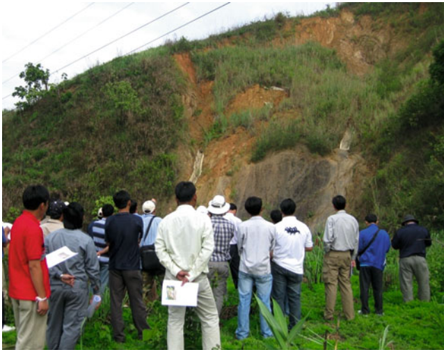
Fig. 2 Trainees at typical site of shallow failure and slope erosion above the road
