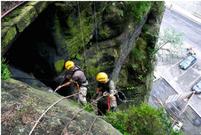
Fig. 1 Monitoring of the rock movement of the sandstone tower near the city of Děčín, Czech Republic. The photo shows also elements endangered by possible rock fall – road and parking lot (Photo by Strix Chomutov, a.s.)
