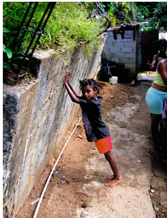
Fig. 2 Retaining wall on a landslide prone hillside, built by a resident in the belief that it would provide sufficient structural support to reduce landslide risk
