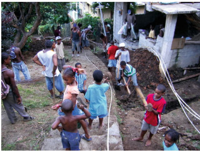
Fig. 2 Action-to-Knowledge (A-K): community residents commencing drainage construction in a vulnerable community in which houses had previously been destroyed by landslides
