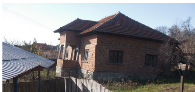
Fig. 4 Photograph of a banded household (2007), located in a sinking area of 2–4 m (see Fig. 1)
