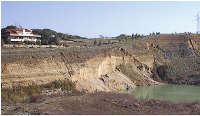
Fig. 1 Example of a large abandoned quarry face for many years in extremely critical condition. The stratigraphy consists of tuffs, sands and gravels with a horizon of clay at the base that supports the aquifer (Rome, Ponte Galeria)
