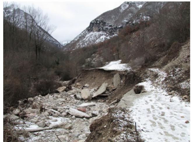
Fig. 5 The bank erosion of the Scura Torrent carried out large part of the morphological terrace cancelling out route and temporarily isolating the locality of "Le Casette"
