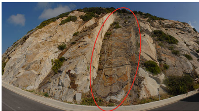
Fig. 7 Plane failure surface along high persistence discontinuity
