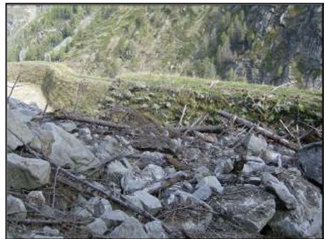
Fig. 15 Embankments built along the SR 47 (291 m and 50 m long) and fill with stones, debris and trees
