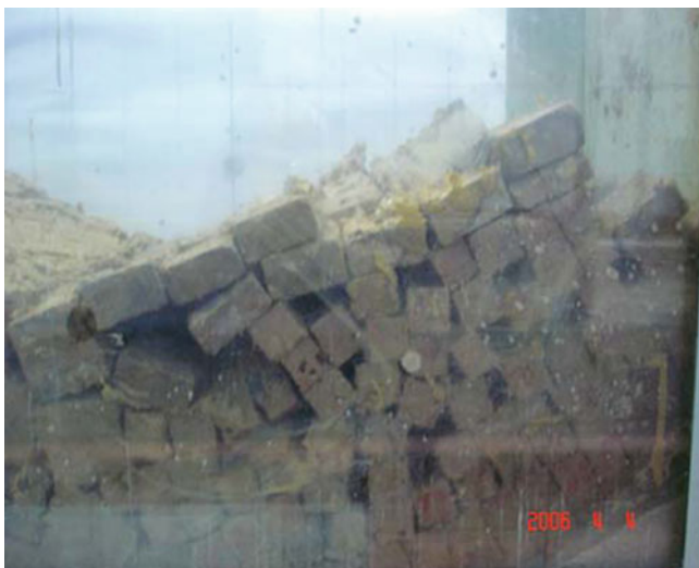
Picture 4 Tension crack and sinking zone occur at the trailing edge of the consequent slope
