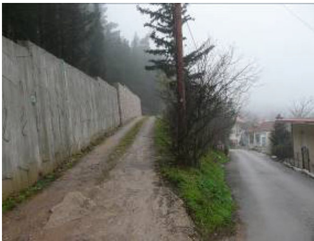
Fig. 2 Barrier constructed in order to reduce the rockfall hazard and in only a part of the slope
