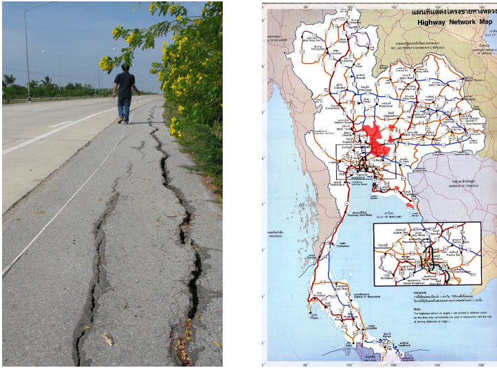
Fig. 1. Longitudinal cracking along pavement shoulder.
