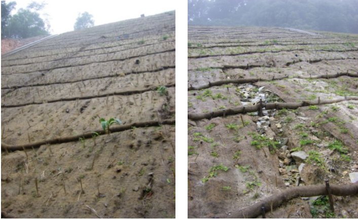
Fig. 10. Test slope with a section (left) covered with natural blanket, and another section (right) covered with natural blanket and plasticity soil.
