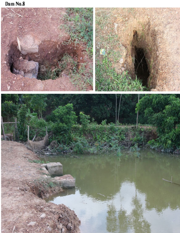
Fig. 29.6 Piping failure resulting from construction or material defects and inappropriately designed spillway
