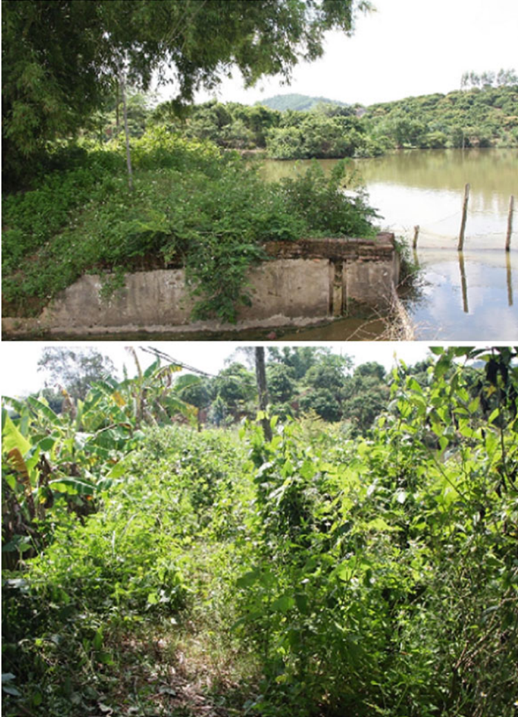
Fig. 29.3 Excessive vegetation and trees on both the upstream and downstream slopes
