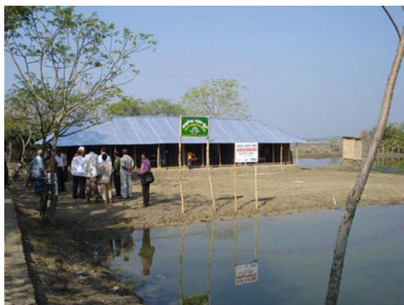
Fig. 15.8 Partially damaged school ( Source Save the Children, 2010)
