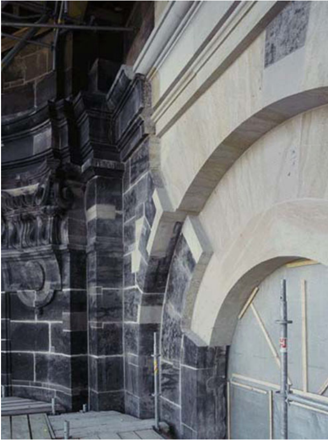
Fig. 6.11 The remaining part of the wall of the destroyed Frauenkirche Dresden and the rebuilt body of the church fit well together. Incompatibilities of old and new material have to be fully excluded in order to ensure the stability of the building
