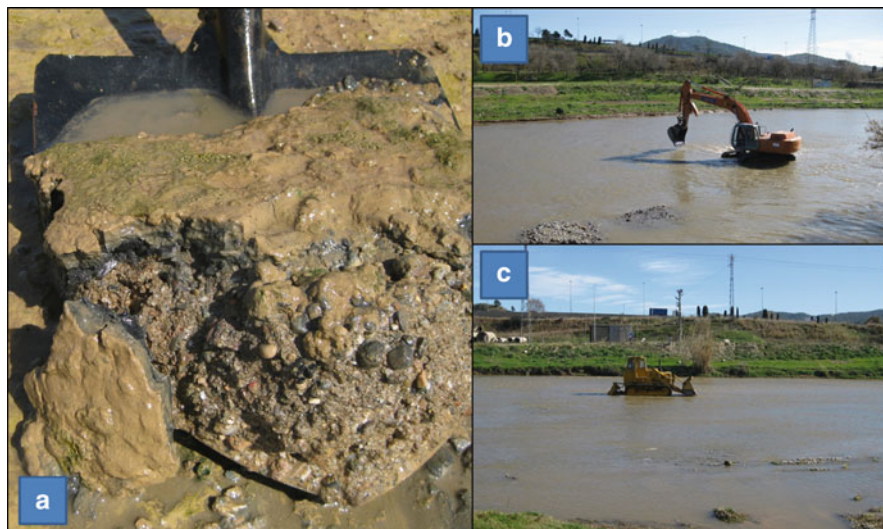
Fig. 2 (a) Close look to the superficial clogging layer before scarification; (b) Machine used first to even the river bottom, allowing for (c) the scrapper (a smaller machine) to perform the actual scarification
