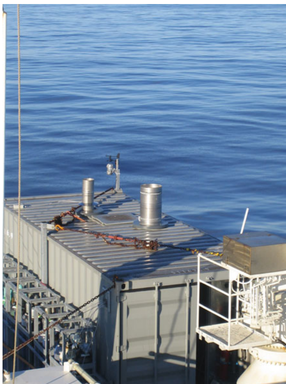
Fig. 17.11 CI-ITMS ship container with two blower inlets on top of the roof aboard the research vessel celtic explorer
