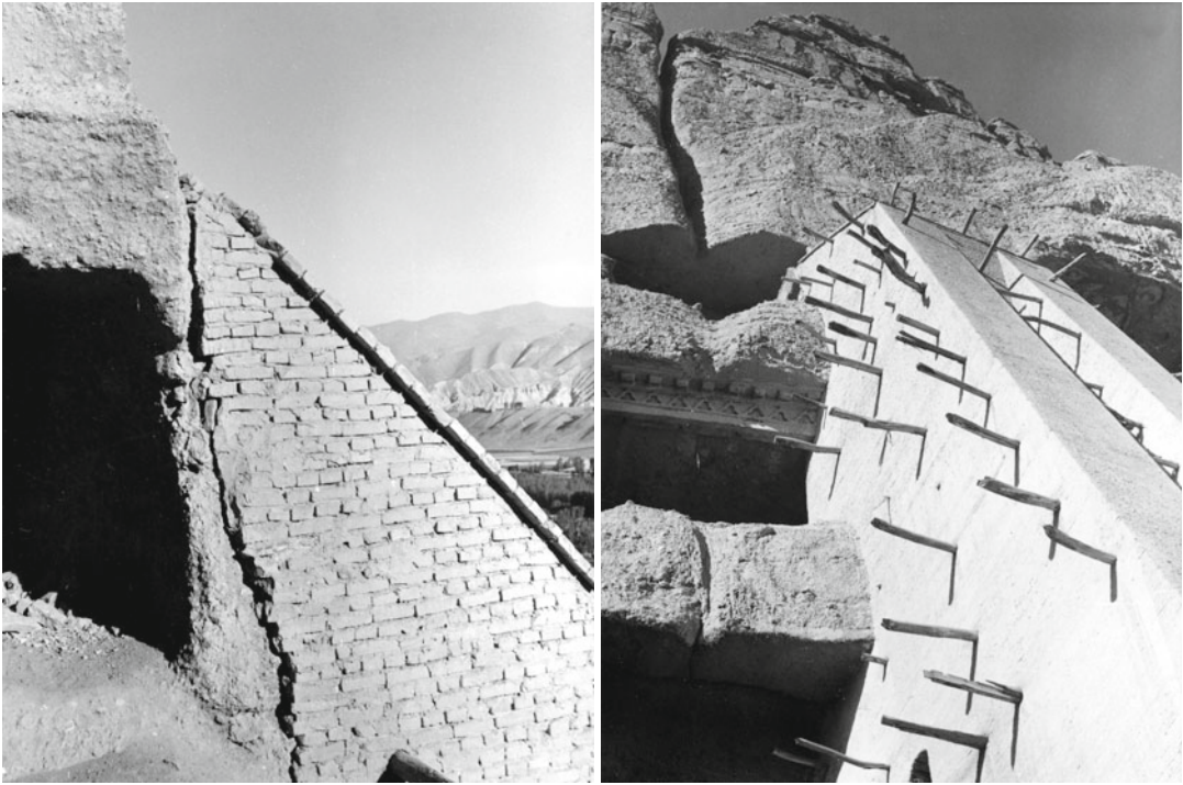
Fig. 9.1 The top of the buttress constructed by the French Archaeological mission (Photos A. Bruno, Sept. 1960)
