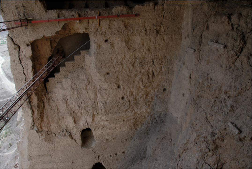
Fig. 12.3 The metallic net protecting from the detachment of small rocks from the shear band of destroyed statue. The photo also shows the wooden spacers, covered
