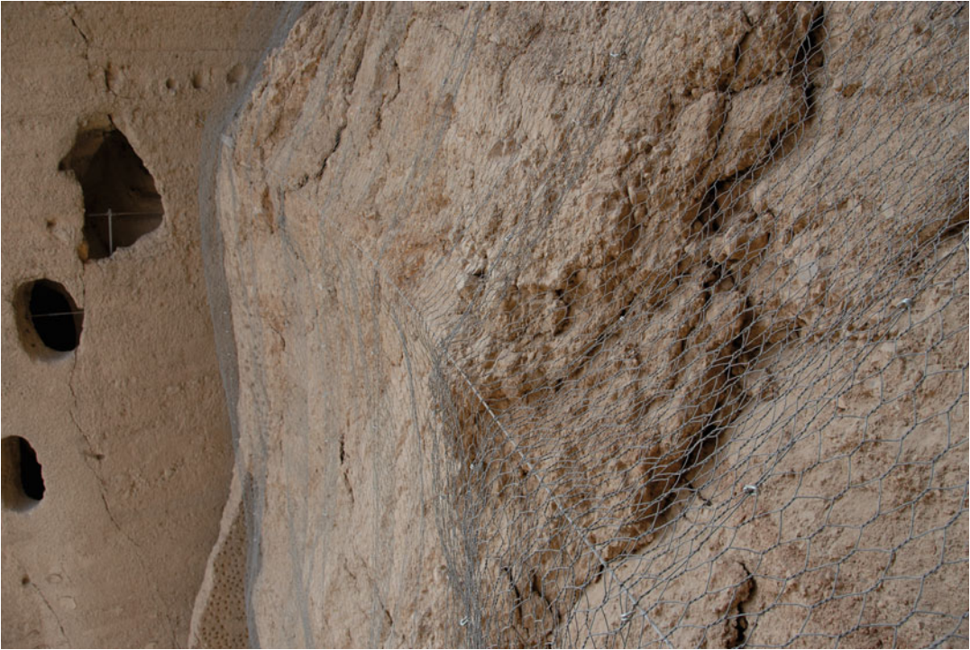
Fig. 12.4 Detail of temporary net and of the shear zone on the back side of Eastern Giant Buddha niche
