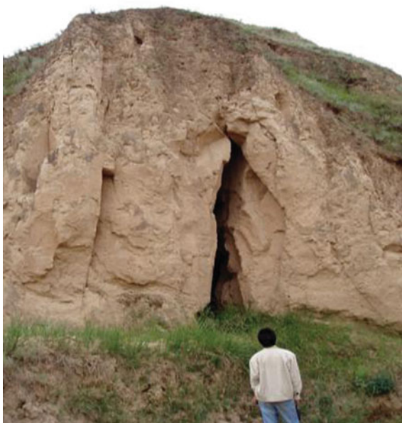
Fig. 11 Erosion along loess joints
