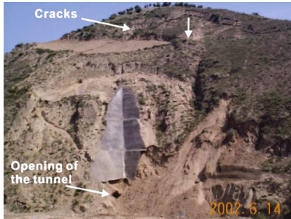
Fig. 24 Collapse and slide occurred in the opening as the tunnel being driven after a heavy rain
