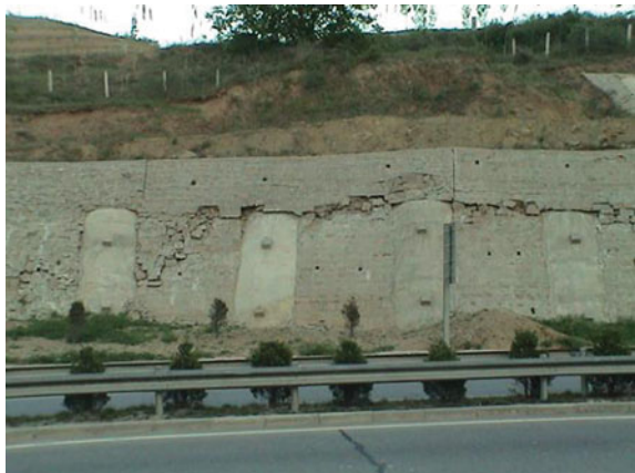
Fig. 28 The damaged beam-anchors for stabilizing the landslide
