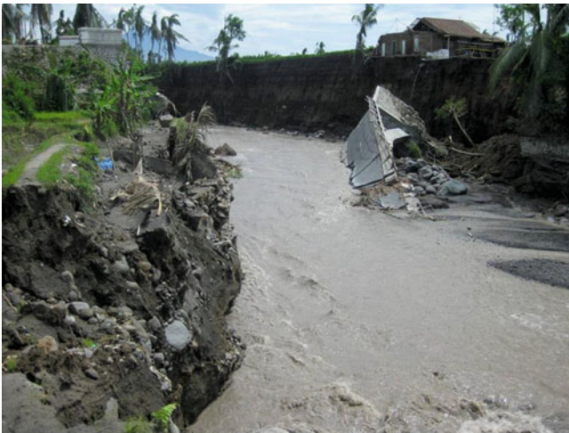
Fig. 2 Collapsed bridge due to the destructive power of rainfall-induced debris flow
