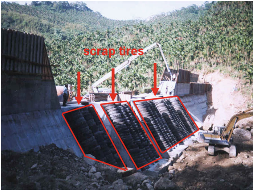
Fig. 12 Slit dam with scrap tires installed to reduce debris flow impact. Huashan River at Kukeng Township of Yunlin County, Taiwan
