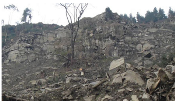
Fig. 3 Unstable rock No. 3
