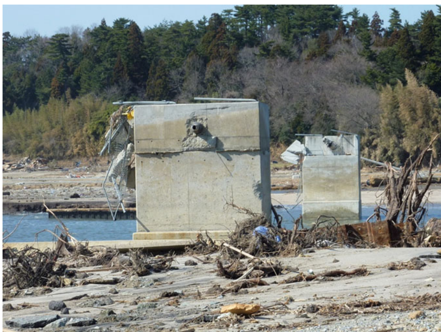
Photo 5 Damage to water pipe bridge
