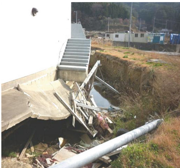
Fig. 11 Scour phenomena around a structure's foundation in a coastal are due to tsunami
