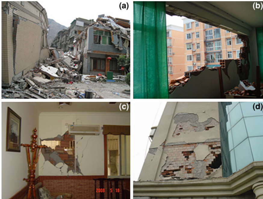
Fig. 8 The damaged infilled walls
