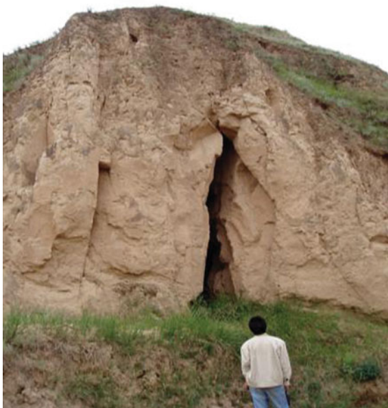
Fig. 11 Erosion along loess joints
