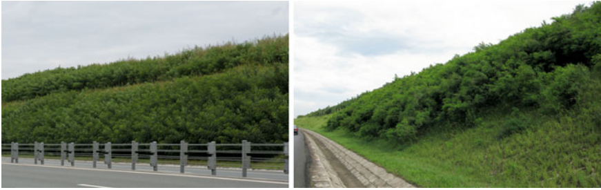
Fig. 4 Highway slope covering with Amorpha fruticosa (AF) ( left ) and Lespedeza (LP) ( right )
