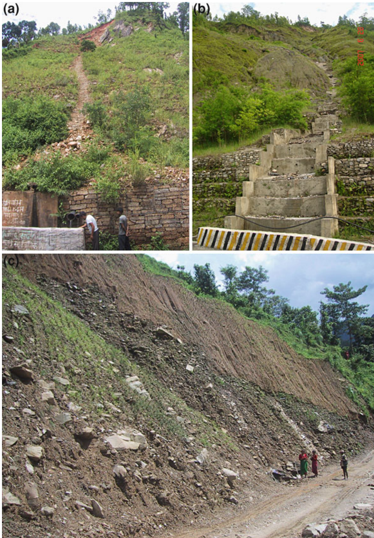
Fig. 21 Bioengineering works to mitigate landslide disaster and applied to various roadside slopes of highways and roads, a French drain and grass plantation in a landslide site of the Arniko Highway, b Drainage measure and tree grass plantation in Krishnabhir landslide (Photo courtesy: Anjan Kumar Dahal), c Coir netting and grass plantation in roadside slope of a rural road
