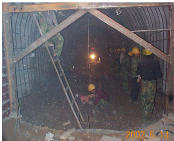
Fig. 25 Steel supports were twisted by deformation of the inner wall of the tunnel
