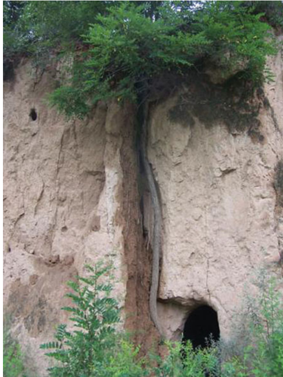
Fig. 18 The flow of rain water along vertical joint in the loess, root also grows along the joint
