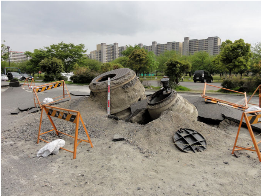
Photo 4 Uplift of underground water tank
