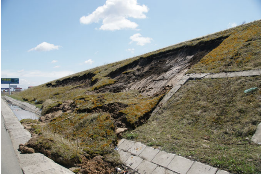
Fig. 1 Shallow slope failure occurred along the Jia-Ha highway
