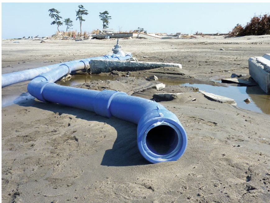
Photo 6 Damage to pipe by scouring of tsunami
