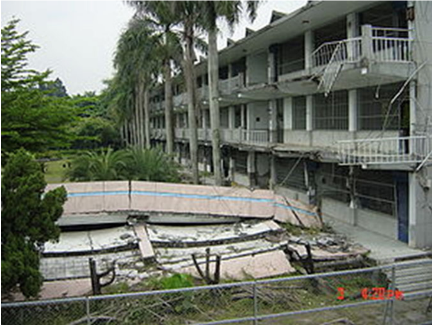
Fig. 4 Heavily damaged Guangfu elementary school in Wufeng (wikipedia: 921 earthquake)
