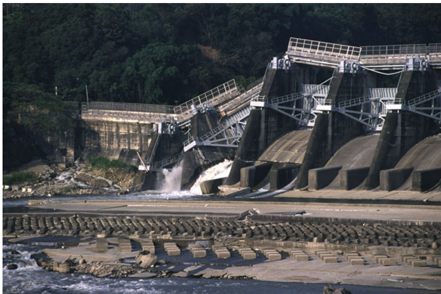
Fig. 5 Damage to Shih-Kang dam
