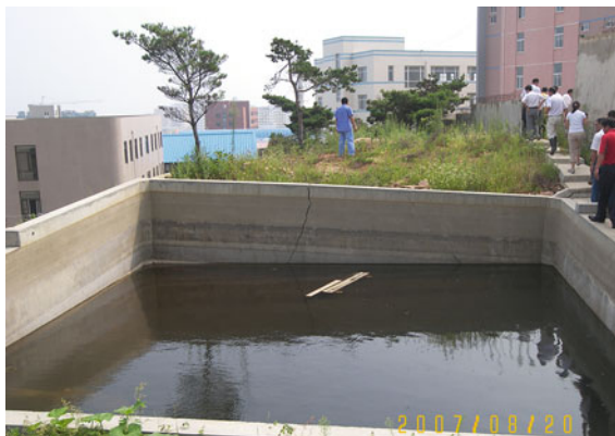
Fig. 2 Incline deformation of impounding reservoir at the end of the slope
