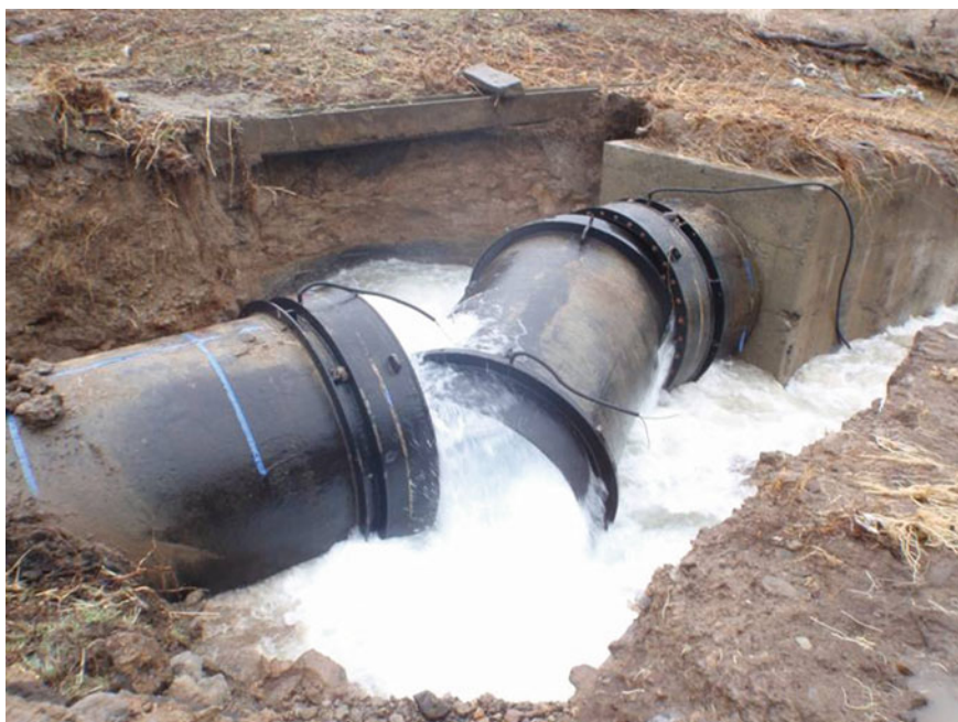
Photo 3 Damage to steel pipe with 2400 mm diameter ( http://www.pref.miyagi.jp/kigyoo/ )
