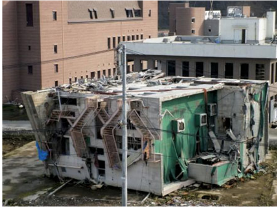
Fig. 5 Overturned building caused by tsunami hydrostatic and hydrodynamic forces in Onagawa
