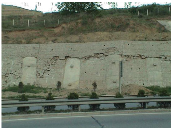
Fig. 28 The damaged beam-anchors for stabilizing the landslide
