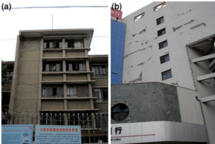
Fig. 11 The damaged irregular buildings, a irregular building in planar direction, b irregular building in planar direction and facade
