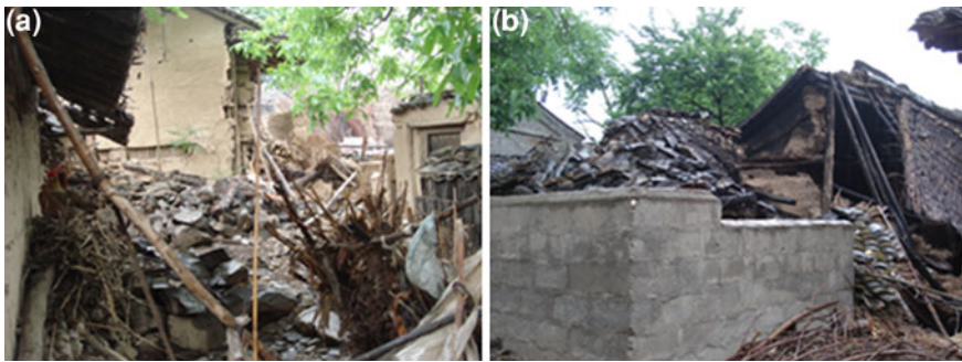
Fig. 3 The collapsed timberwork buildings
