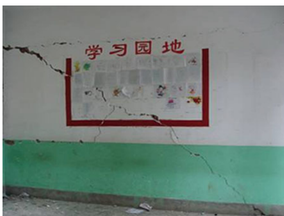
Fig. 14 The diagonal cracks of cross wall
