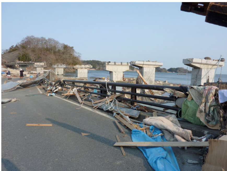
Photo 2 Damage to bridge by tsunami
