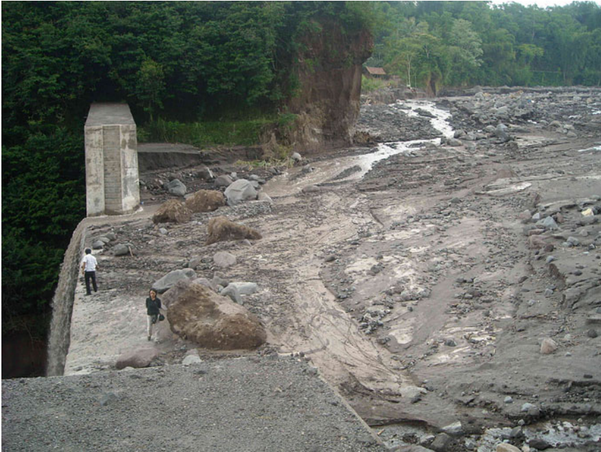
Fig. 5 Upstream condition of Boyong River: Sabo dam BOD4 on 14 January 2011
