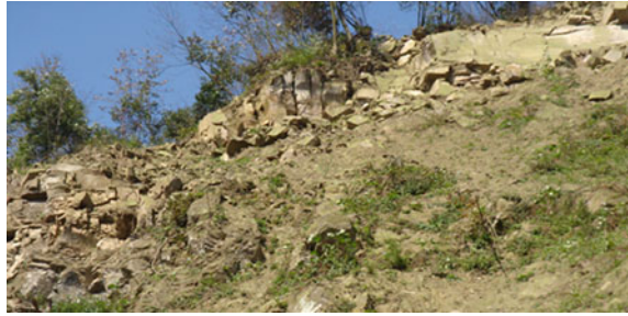
Fig. 1 Unstable rock No. 1
