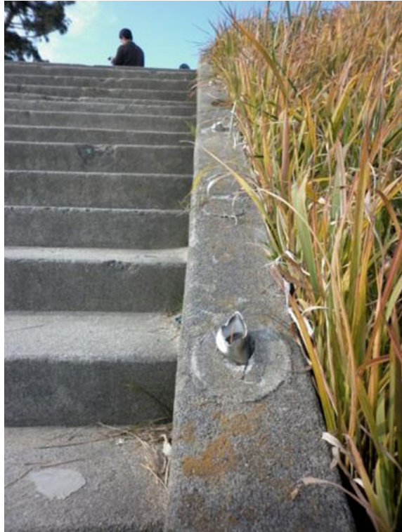
Fig. 9 The broken handrail remains in the footsteps of the overtopped high ground level designed for vertical evacuation facilities due to the March 11, 2011 tsunami
