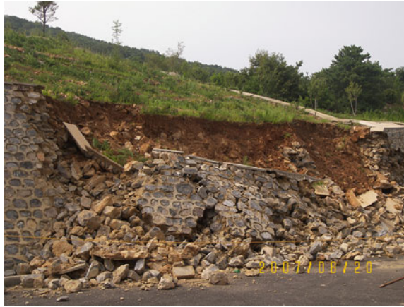
Fig. 1 Loose accretion at the front of the slope
