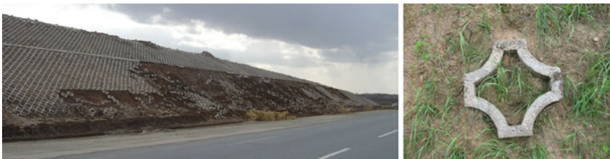
Fig. 3 Slope failure in Jia-Ha highway protected by hollow blocks
