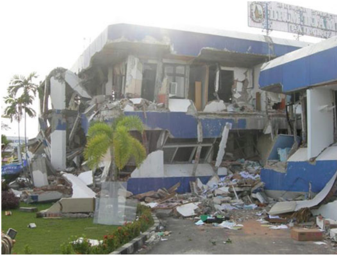
Fig. 13 An example of a vulnerable building during September 30, 2009 Padang earthquake that shall not be assigned as tsunami vertical evacuation structures
