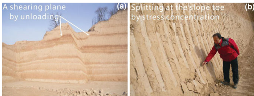
Fig. 23 A new excavated building site located in Longshou village, Huanglin County, Shaanxi. The west side has a shearing plane at the top by unloading (a); the toe of the north side was spited to slices by the concentrated stress (b)
