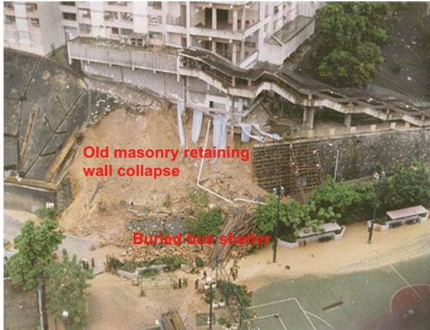
Fig. 8 Collapse of Kwun Long Lau old masonry retaining wall in 1994 (modified after GEO)
