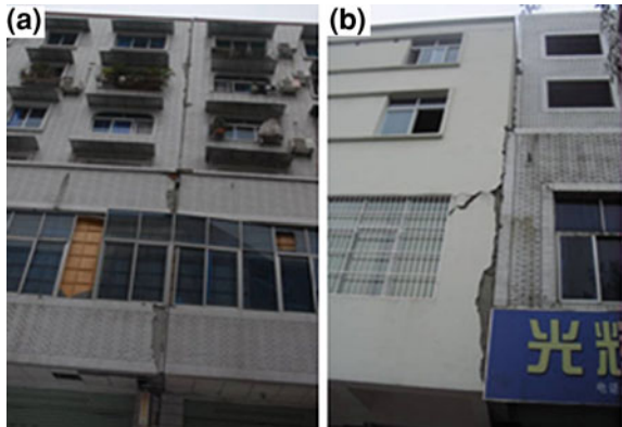
Fig. 7 The damaged buildings without aseismic joints
