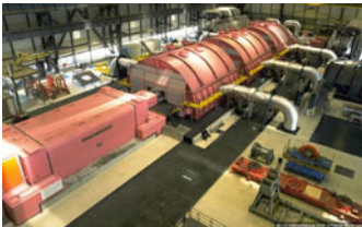
Fig. 1 Alternator in power plant
