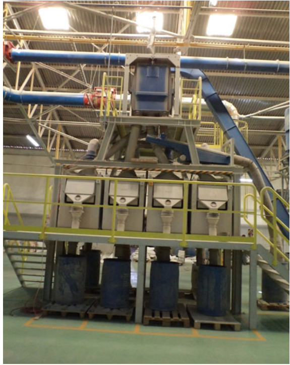
Fig. 4.17 Vibratory screen with electro static separator and collection mechanism in a WEEE processing unit
