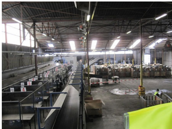
Fig. 4.12 Waste segregation facility with provision for hand sorting
