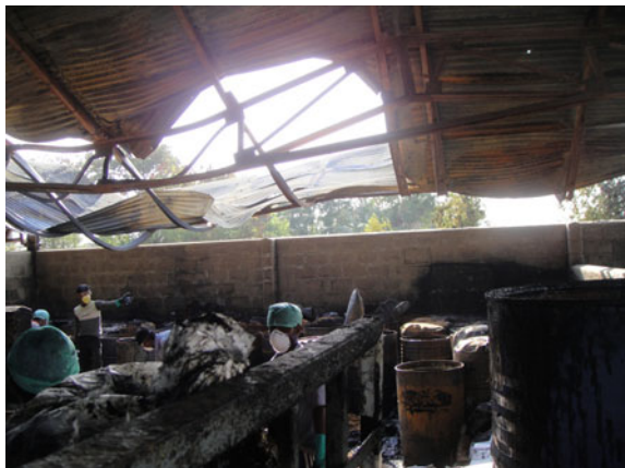
Fig. 13.15 Partially damaged structure during a fire accident
