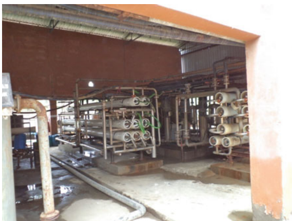
Fig. 10.3 Reverse osmosis plant
