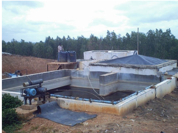
Fig. 5.6 Leachate treatment facility
