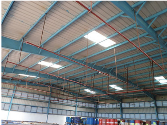
Fig. 11.12 Sprinkler system in hazardous waste TSDF
