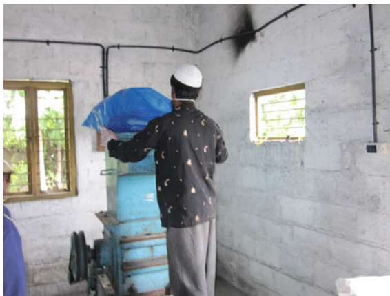
Fig. 6.14 Biomedical waste being fed into the shredder
