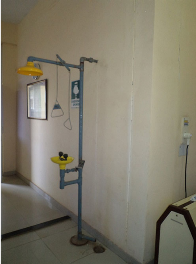
Fig. 11.13 Emergency shower and eyewash in hazardous waste TSDF
