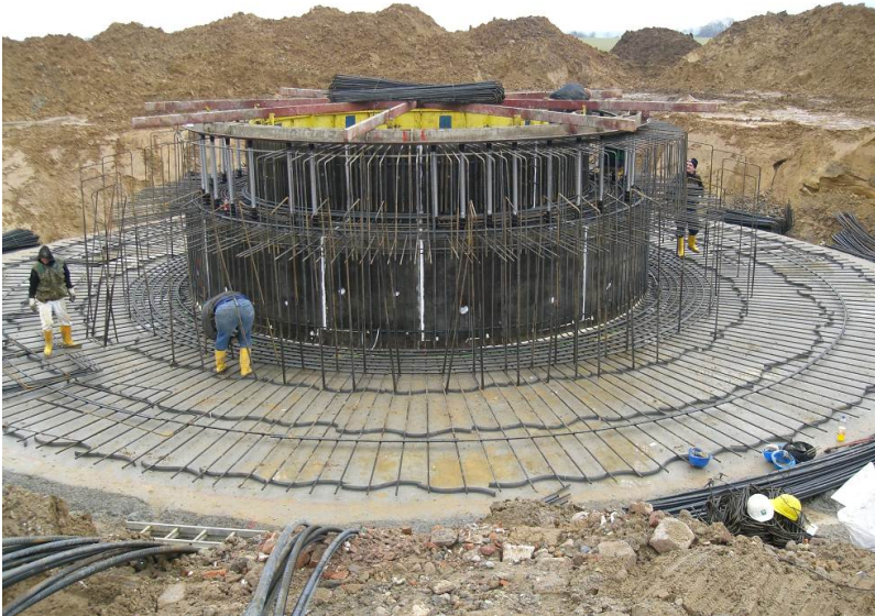
Fig. 12.35. Construction of the foundation and integrating the foundation section of the tower
