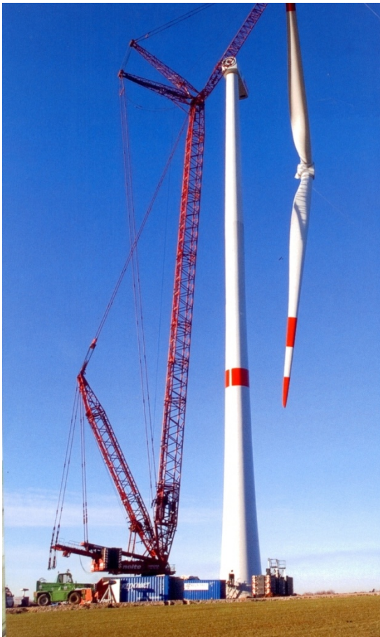
Fig. 12.27. Hybrid tower of a Repower 3.4 MW wind turbine, height 123 m (Max Bögl Group)
