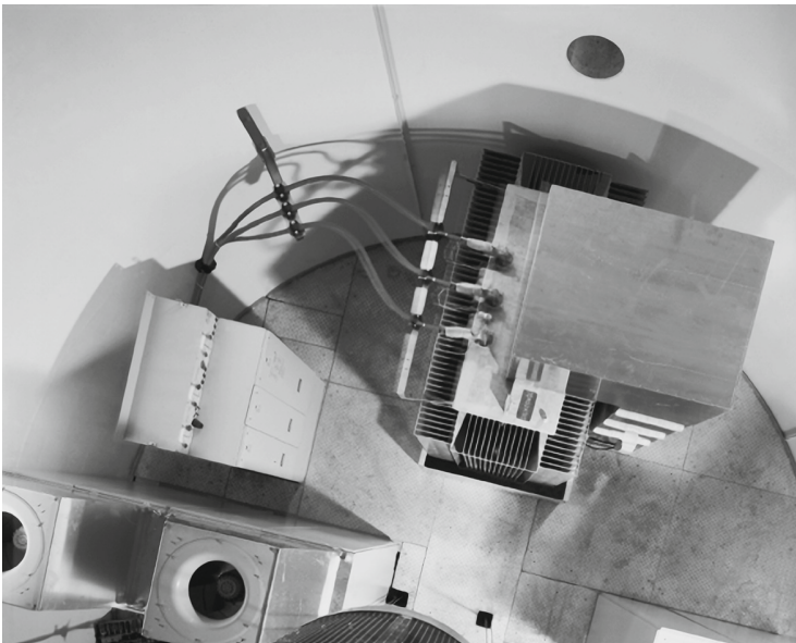
Fig. 12.17. Installation of the transformer and of the SF-6 switchgear in the tower base (Enercon)
