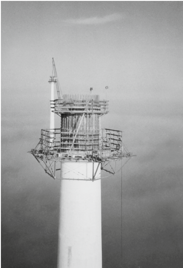
Fig. 12.22. Construction of a tower for an Enercon E-66 with site-mixed concrete (Enercon)
