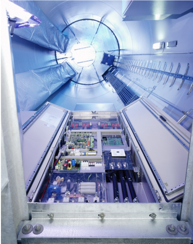
Fig. 10.26. IGBT inverter, 2 MW rated power, in the tower of an ENERCON turbine (Enercon)
