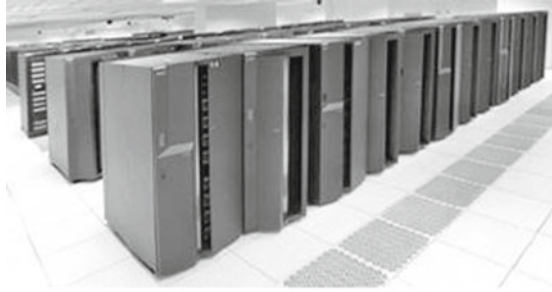
Fig. 16.24 Top: ASC Purple installation at Lawrence Livermore National Laboratory (photo courtesy of LLNL), bottom: rear view on ASC Purple rack showing the optical fibers [79] (© 2005 IEEE)
