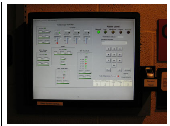
Fig. 10. Operator Information and Control Touch-Screen Panel
