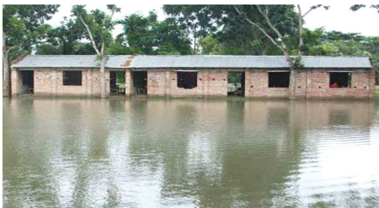
Fig. 13 An affected secondary school in Keshabpur Upazilla . Source: (Khan 2008)
