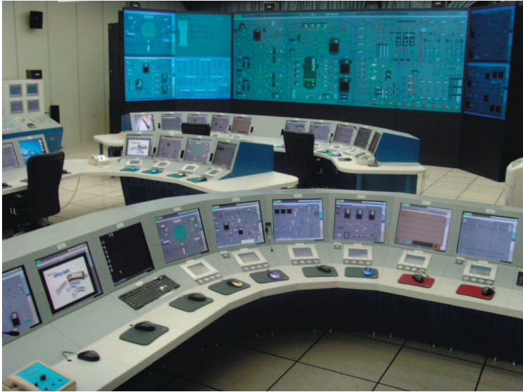
Fig. 1. Main control room of APR1400 [7]
