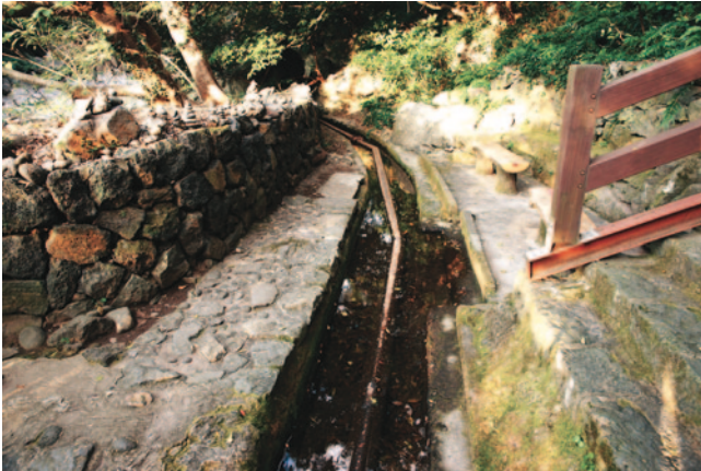
Fig. 6.47 A part of Cheonjeyeon irrigation canal system built in the early 20th century
