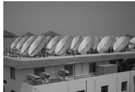
Figure 3: Installed Scheffler Concentrators, Project from 2008/09
