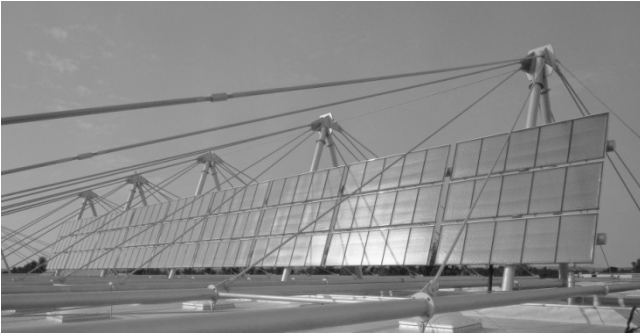
Figure 3: Solar collectors on top of the Solvis plant
