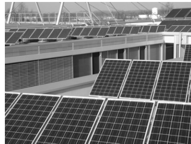
Figure 2: Solar collectors above the atrium
