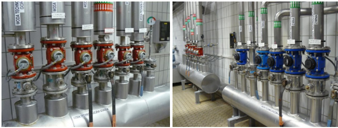
Fig. 5. Water measuring systems
