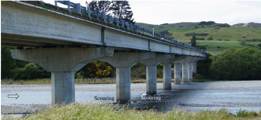
Fig. 10.18 Scour taking place at bridge piers in a field condition. Photograph by the author
