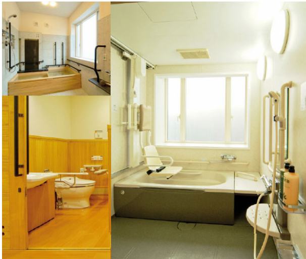
Fig. 9. Modular Buildings are fully equipped with assistance technologies in the factory. Sekisui Heim.
