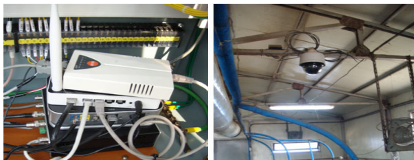
Fig. 3. DVR and CCTV camera
