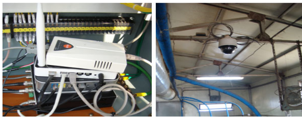
Fig. 3. DVR and CCTV camera
