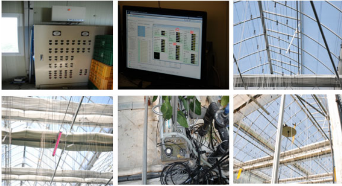
Fig. 10. PLC controller and Greenhouse Facilities
