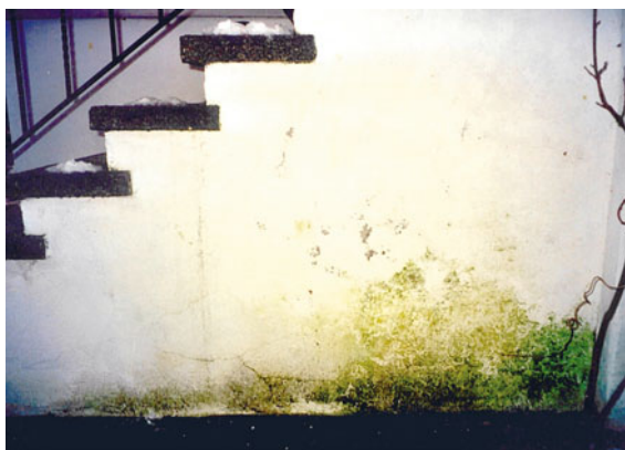
Fig. 14.19 Growth of algae on a painted facade
