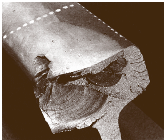
Fig. 16.27 Broken rail caused by head checks
