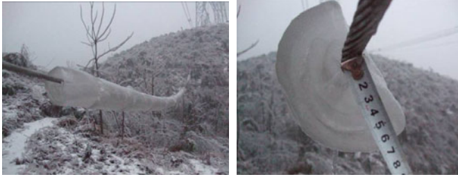
Fig. 1. Condition of Icing on Ground Wires
