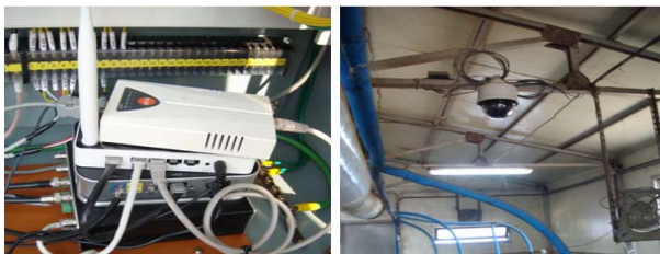
Fig. 3. DVR and CCTV camera
