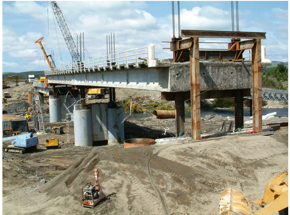
Fig. 12.28 The road bridge at Tangiwai in the process of being raised 2 m and strengthened prior to the 2007 breakout lahar from Ruapehu. Photo Harry Keys
