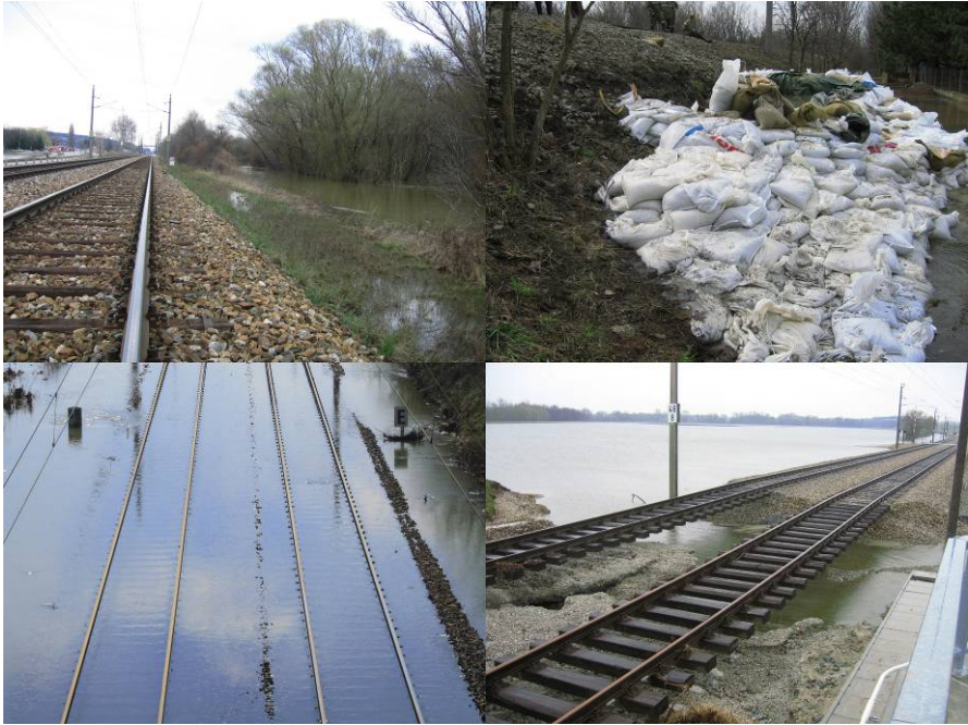
Fig. 1 Field examples of damage grades 1 to 4 to railway lines caused by flooding of the Austrian Northern Railway line by the March River in April 2006. Photos provided by ÖBB-Infrastruktur AG.
