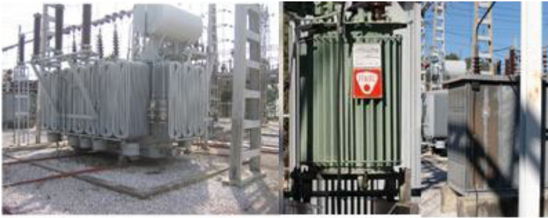
Fig. 2. Protected substation components: HV/MV Power Transformer (left), Neutral Reactance (centre) and Neutral Resistor (right)
