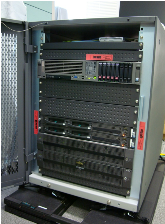
Fig. 1. The WISE-CAPS servers (two servers in the center of the rack) and an attached storage (the bottom of the rack)
