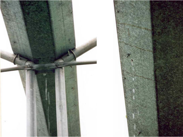
Fig. 8.13 Leaky gutter connection, bare holes or rusted-through holes cause water penetration into the greenhouse, flooding, and destruction of the crop
