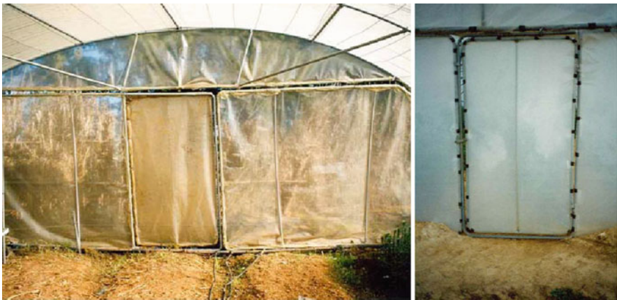
Fig. 8.28 Leaky doors where insects can penetrate and heat energy will be lost at night
