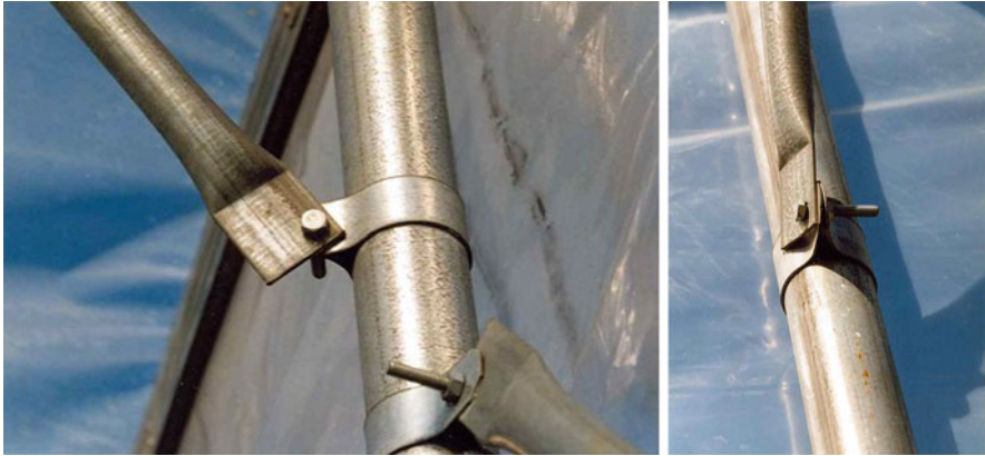
Fig. 8.7 The clamps are screwed tightly together, but the borehole in the brace is near the edge, so that the brace cannot be fastened firmly to the clamp. It is better to bevel the brace and to bore the hole in the middle
