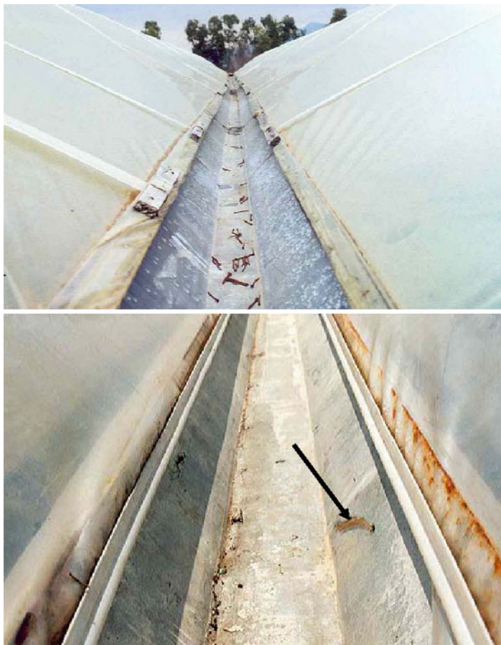
Fig. 8.29 Forgotten nails and screws cause rusting-through of the gutter. One corroded hole is closed by a wooden stopper
