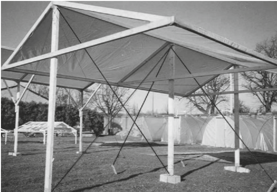
Fig. 5.79 Umbrella-type for terrace shelter structures, fastened by tension wires and earth anchor. The rainwater can be collected by a plastic film gutter dug into the soil. The plastic film is stretched over the structure and fastened at the edges by self-made clips from PVC water tubes cut open in longitudinal direction
