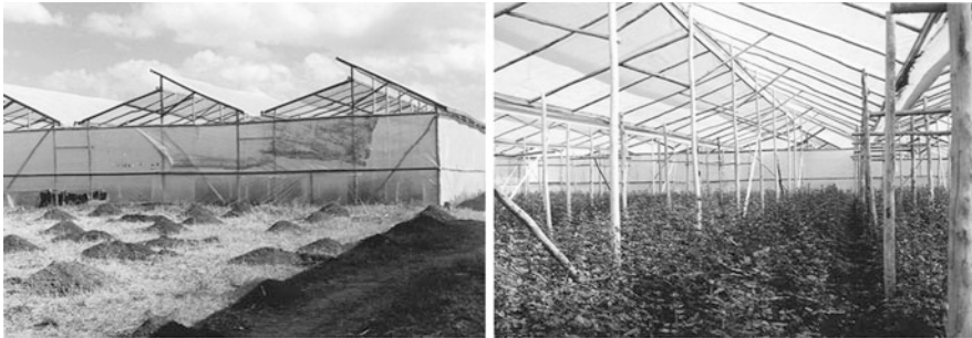
Fig. 5.37 Greenhouse for roses in Malawi with open space only in the roof and gable area, to protect the flowers from wind and sloping rainfall
