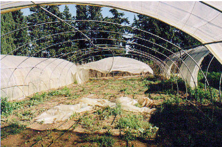
Fig. 4.1 Too weak tunnel structure damaged by wind
