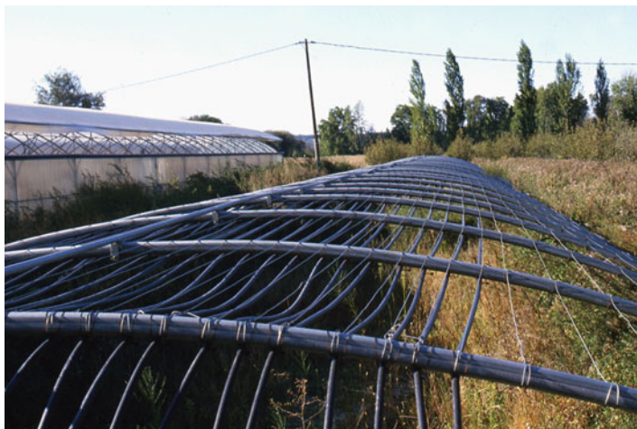
Fig. 12.15 Corrugated PP tubes outside the greenhouse for cooling the geothermal water, when no heating is necessary, Tunisia
