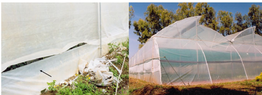
Fig. 10.15 The insect screens are not fixed tightly enough to the structure, so that leaks occur and pest insects can penetrate
