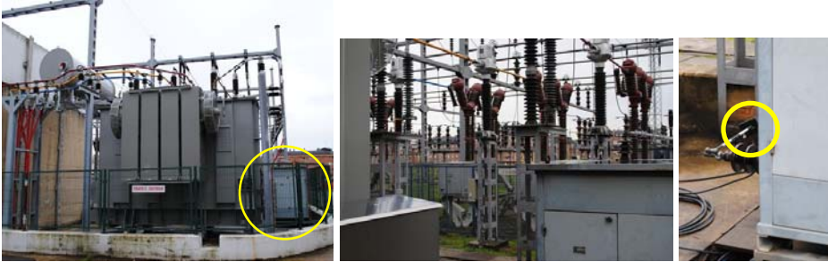
Fig. 1. La Corredoria substation transformer and its NGR (left part). Detail of the connection between the NGR and the neutral (center) and ground (right), showing the current transformer used in this paper.
