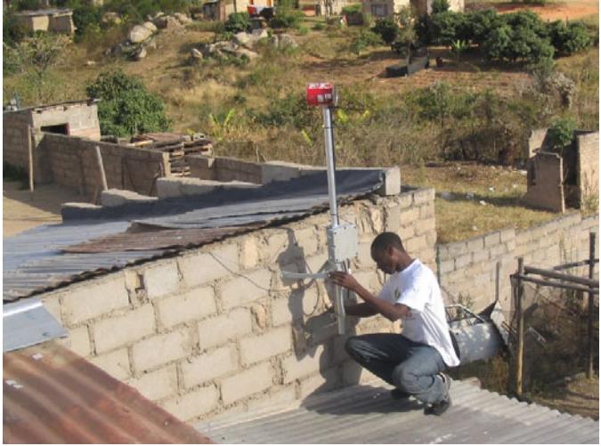
Fig. 4. Installation of a DIY kit for wireless communications, provided by the Meraka Institute of CSIR
