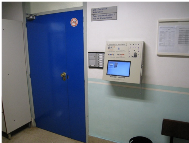
Fig. 7. Physical installation (at EUPMt) in a wall for door opening system
