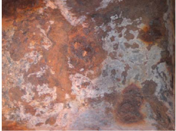
Fig. 3 Surface rust of the nut
