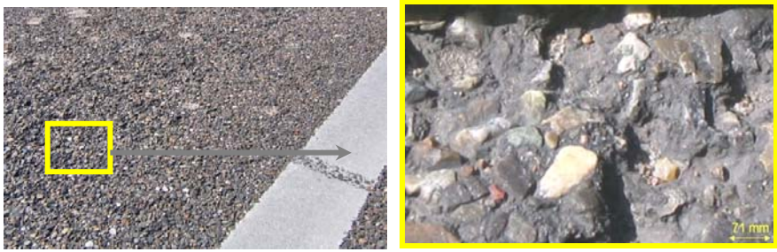
Fig. 12. Raveling of porous asphalt concrete (left) means that the pavement surface loses aggregate particles (right).
