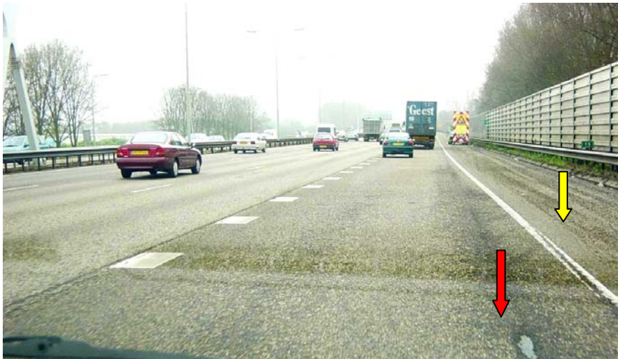
Fig. 13. Raveling of porous asphalt concrete on a Dutch motorway.
