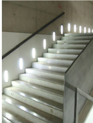
Fig. 6. Escape lighting for staircases.
