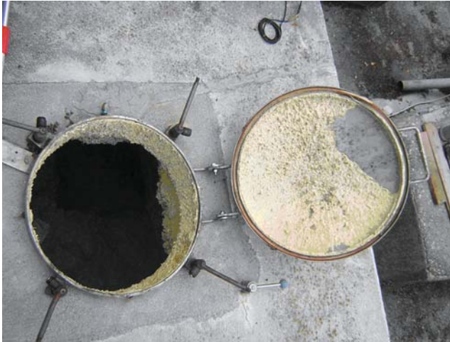
Fig. 4.6 Surface of gas-dome and manhole cover of an agricultural biogas plant coated by precipitated elemental sulfur from biological H_2S oxidation (Foto: F. Wackerle)
