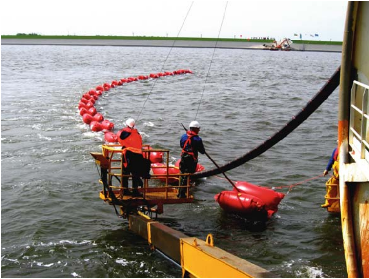
Fig. 7.15 Floating of a submarine power cable during landing (NorNed). Crew members wear safety harness
