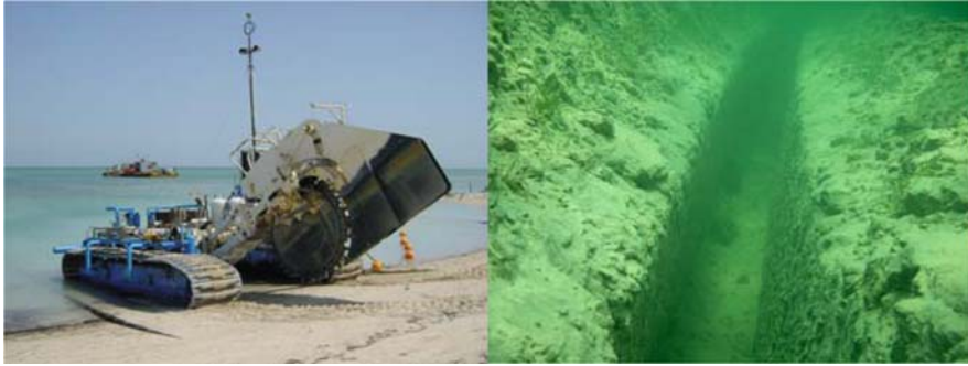
Fig. 7.26 Wheel cutter for rocky seafloor. Cable trench cut into calcarite seafloor (Courtesy of LD Travocean, France)
