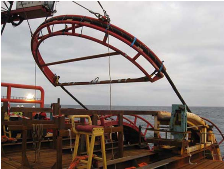
Fig. 7.18 The quadrant, a steel support frame, goes into the water (Courtesy of ABB, Sweden)
