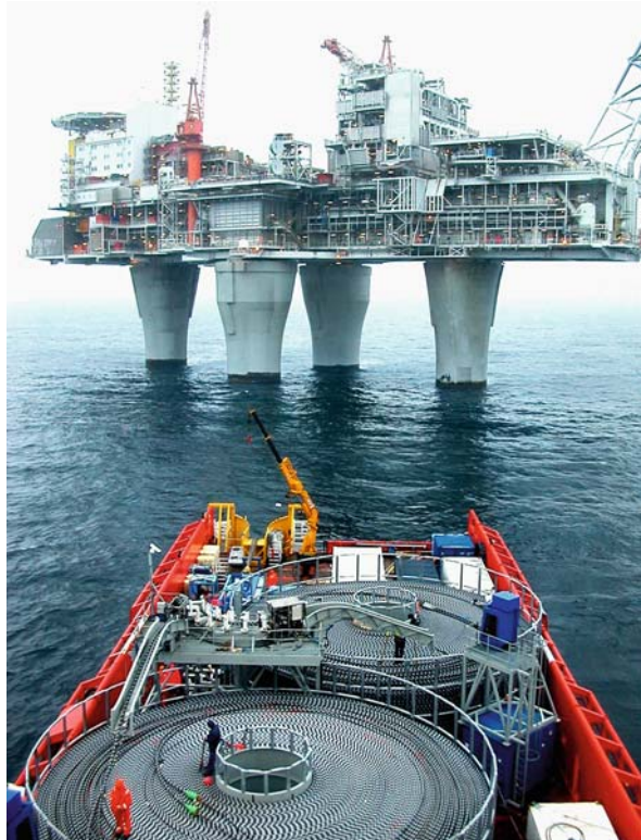
Fig. 1.3 The Norwegian gas platform “Troll A” receives its electric power supply from a pair of HVDC cables (Courtesy of ABB, Sweden)
